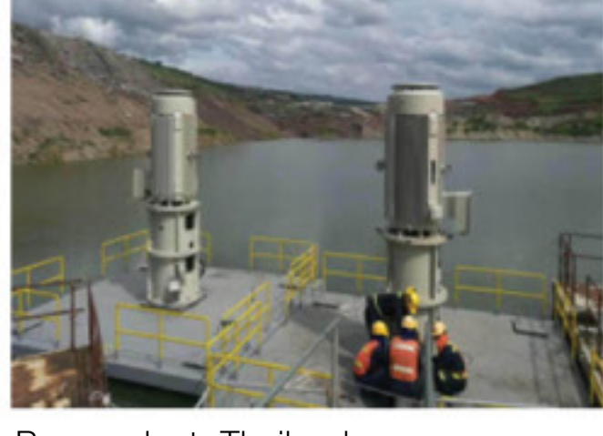
Power plant, Thailand
