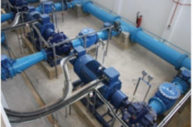
Water plant, Malaysia
